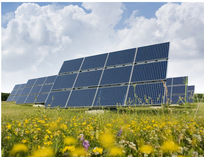
Solar panels capture the sun's rays at a solar power plant.
